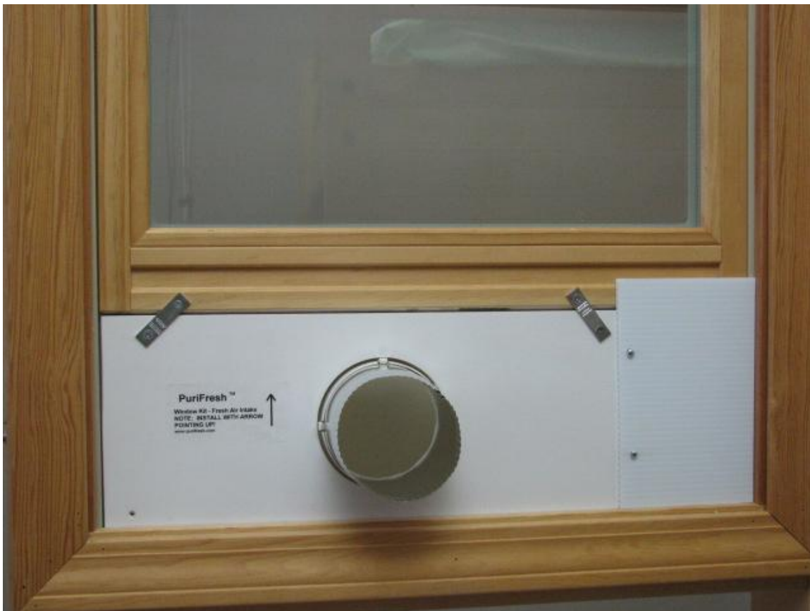
Figure 4: Cut a corrugated plastic piece to cover the opening on the side, with a 1-inch overlap, then attach it to the Fresh Air Intake with two of the round head wood screws, as shown.
