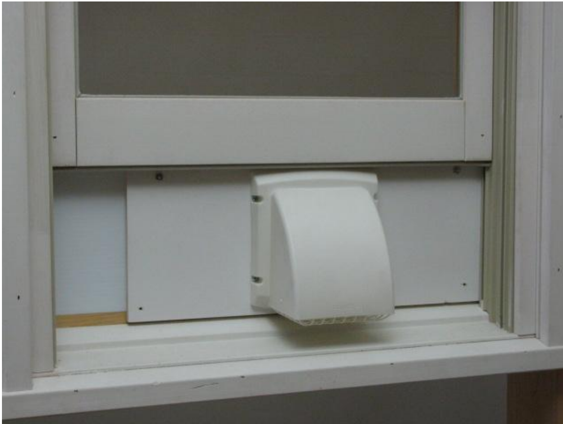
Figure 6: Outside view of the fresh air intake after installation in a window.
